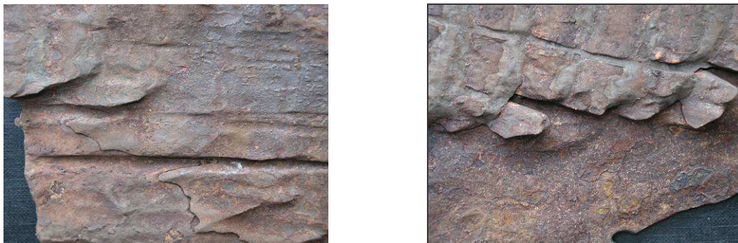
Figure 4. A view of strongly eroded, corroded and cracked surfaces of 4666 CDP deposit and CORTEN steel fan body, 2x magnification
